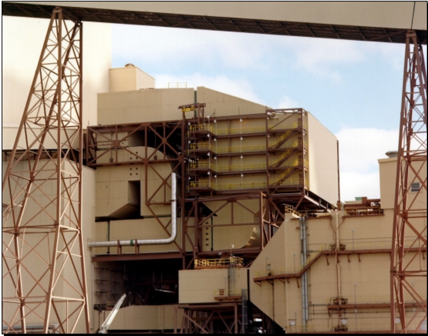
Figure 2: AES Somerset – 675 MW SCR
