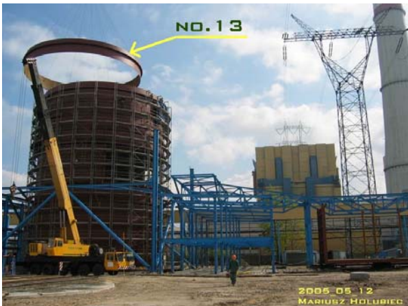
Absorber Assembly – Kozenice - Poland – 800 MW Commercial Operation 2007
