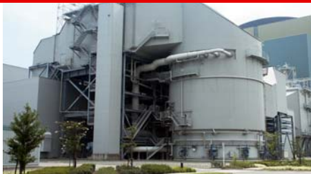
J-Power - Tachibanawan – 1050 MW – Operation 2001
