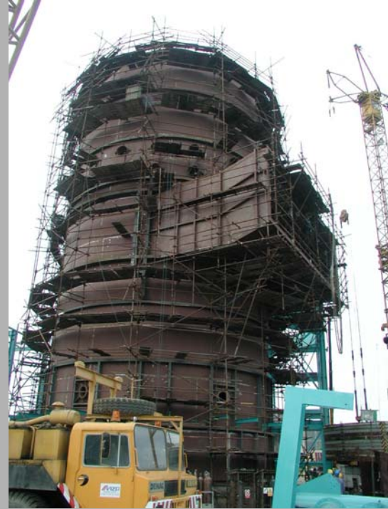
Absorber – Sokolovska Uhelna – Vresova - Czech Republic – 1 Single FGD for 4 x 55 MW Lignite Boilers Commercial Operation 2002
