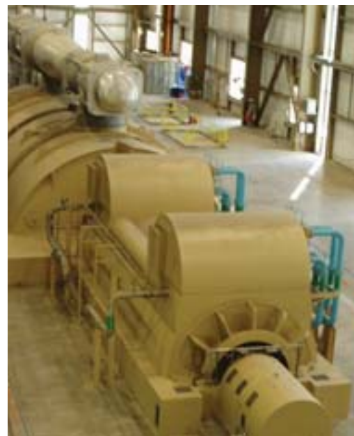
AC generator for MidAmerican Energy Walter Scott, Jr. Energy Center (USA) Capacity: 1,025MVA Put into service: 2007
