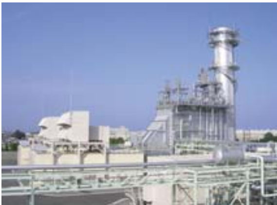
Hitachi, Rinkai combined cycle plant (Japan)
