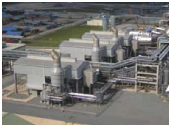
Betara Complex Development Project motor driven compressor drive (Indonesia)
