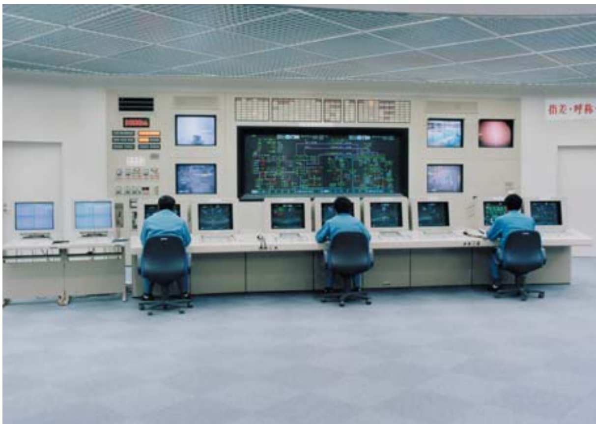
Central control equipment for 1,000MW coal-fired thermal power plant.
