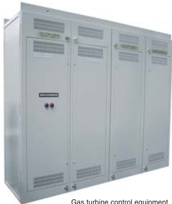
Gas turbine control equipment.
