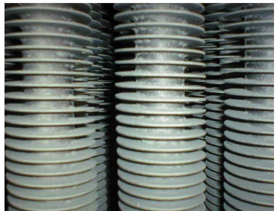
Figure-10 The state of the heating tubes (After 2 years of operation)
